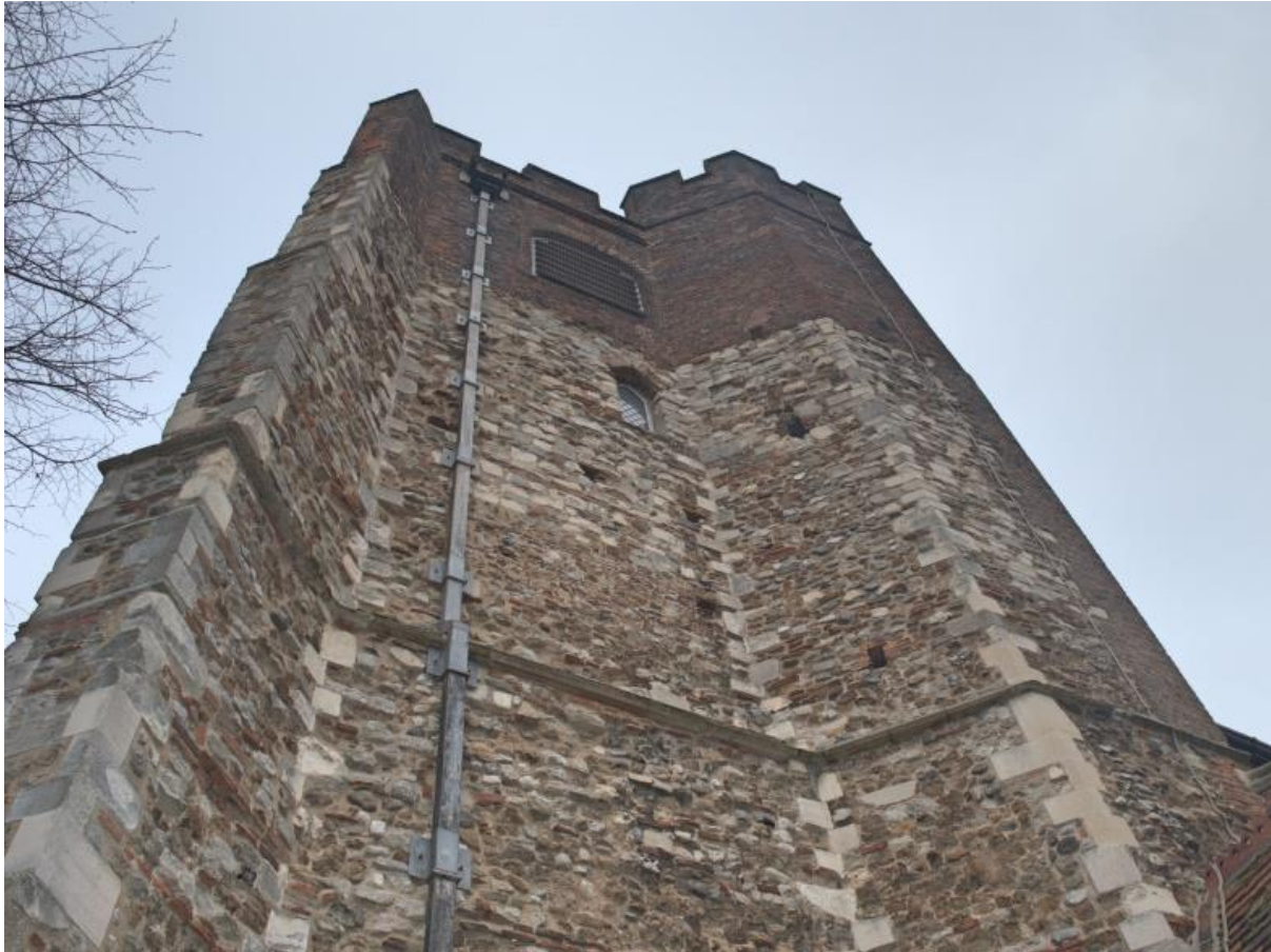
Figure 7: St Mary at the Wall. Note the different brick at the top which shows the eighteenth-century repairs (Picture: author's own).
