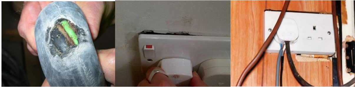
Examples of unsafe electrical plugs, sockets and leads
