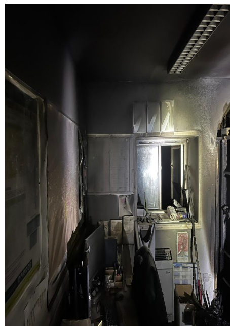
Fire damaged office
