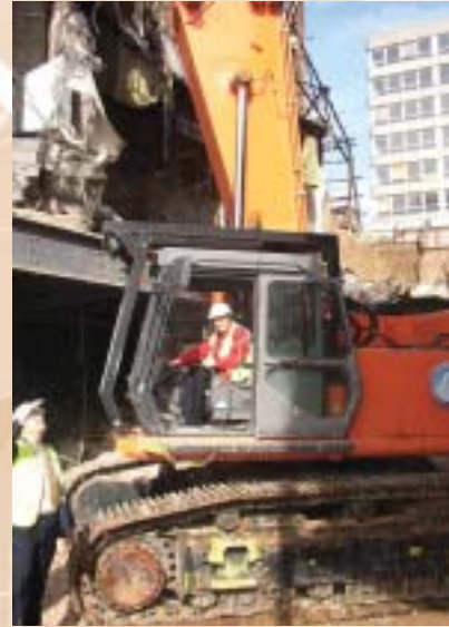
The University's Development Director in Southend, Linda Jones, helps with the demolition of the derelict Odeon cinema. The Prudential building can be seen in the background
